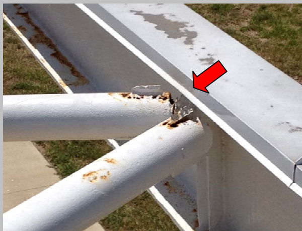
Photo #17 Corrosion of west side central canopy members.
