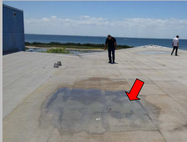
Photo #9 Evidence of ponding at central canopy/main lobby area.
