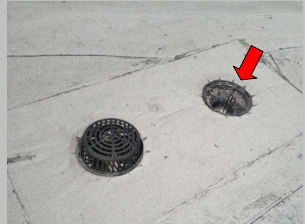
Photo #12 Secondary drain dome missing.
