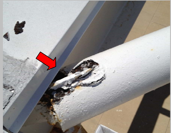
Photo #16 Corrosion of west side central canopy members.
