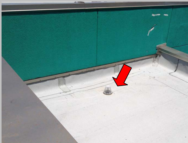
Photo #5 No secondary drainage; puncture of EIFS exterior near Exhibit Storage entrance.
