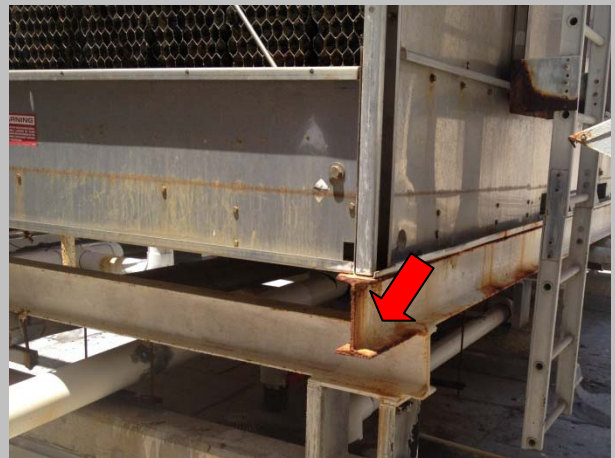
Photo #6 Moderate to severe corrosion at support of mechanical unit located at the Exterior Mechanical Area.
