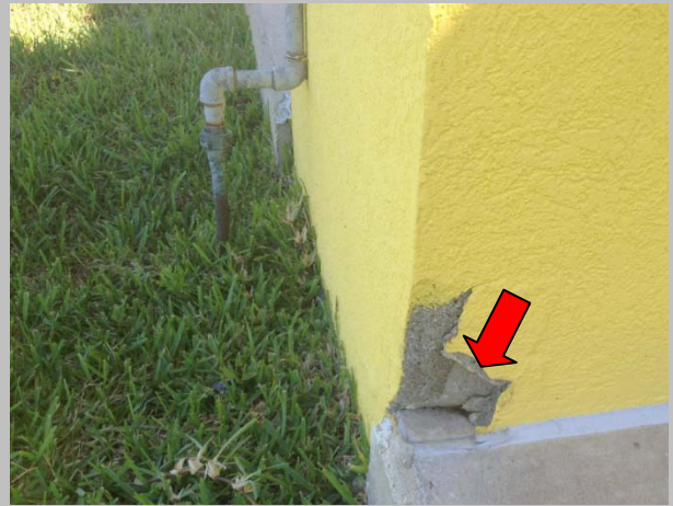
Photo #2 Column base crack at west side walkway.
