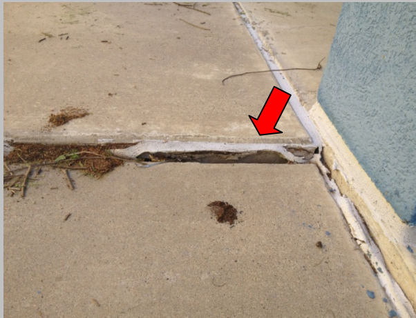
Photo #3 Separation of expansion joint at west side walkway and building slab.
