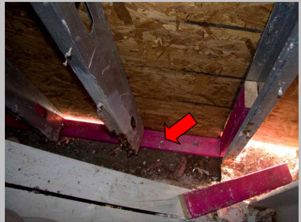
Photo #18 Corrosion at bottom of exterior wall metal studs and track at northeast side of facility. Photo provided by ROFA.
