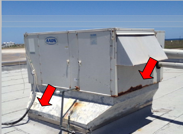
Photo #13 Moderate corrosion of mechanical equipment. Adapter roof curbs at base of mechanical equipment.
