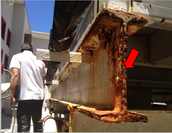
Photo #7 Loss of fasteners and sever corrosion of support of mechanical unit located at the Exterior Mechanical Room.
