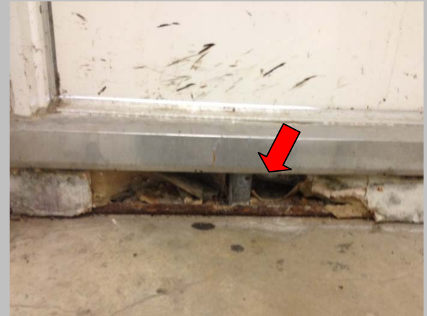
Photo #10 Degradation of sheet rock and metal studs below door to cooling tower.
