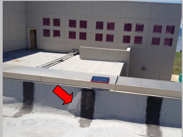
Photo #4 Blistering of cap sheet at base of flashing near Exhibit Hall and Loading Area.
