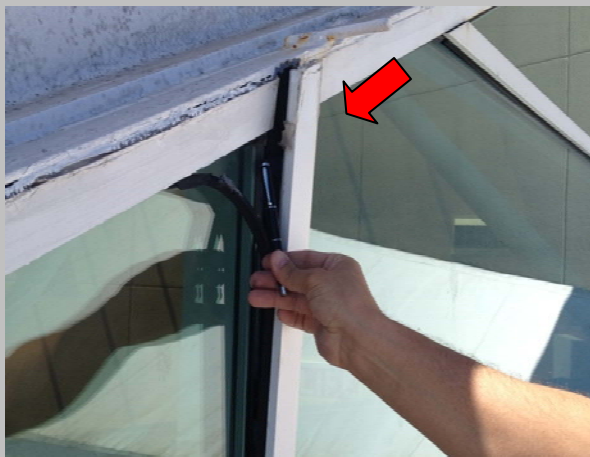
Photo #11 Failure of sealant and loss of mullion at aluminum window at central canopy/main lobby area clerestory windows.
