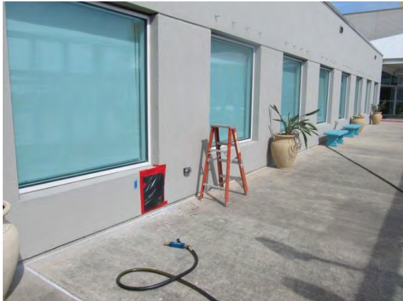
Photo #1 Water spray test near DTO #1.
