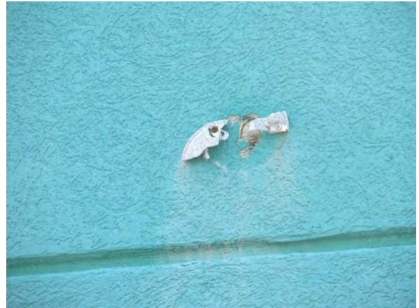
Photo #28 Detail view of damaged referenced in previous photograph.
