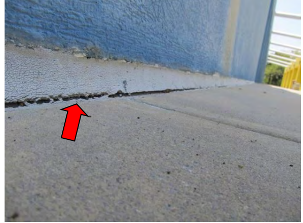
Photo #50 Sealant adhesion failure along bottom of EIFS termination, typical condition throughout.
