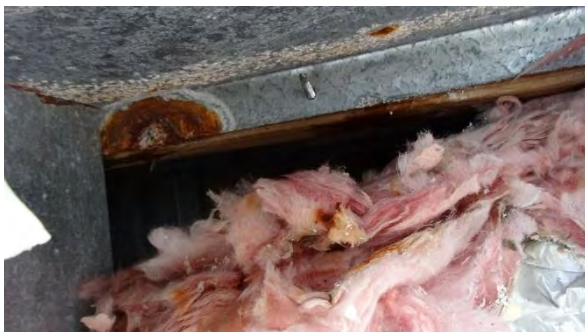
Photo #5 Bottom of window sill. Water was observed on sill pan and wood blocking.
