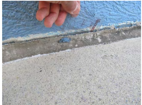
Photo #46 Typical sealant adhesion failure along bottom of EIFS wall termination.
