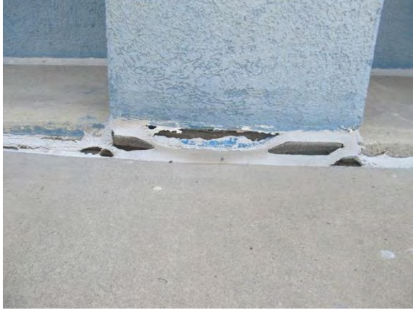
Photo #49 Sealant failure at bottom of EIFS termination, typical condition.
