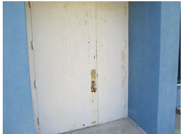
Photo #48 Typical rust on service doors.
