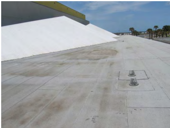
Photo #71 Staining on lobby roof facing east.
