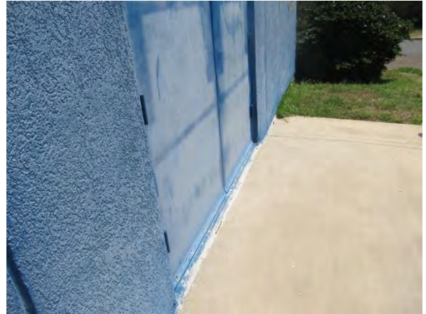
Photo #56 Typical deteriorated and weathered sealant at bottom of doors.
