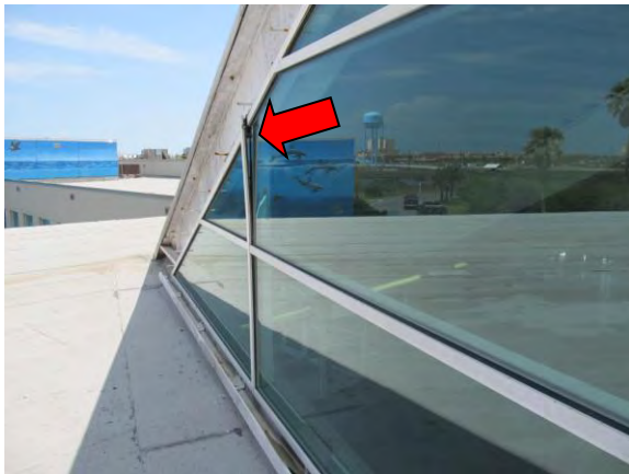
Photo #75 Window system on upper level east elevation adjacent to sloped glazing system. Note displaced vertical mullion.
