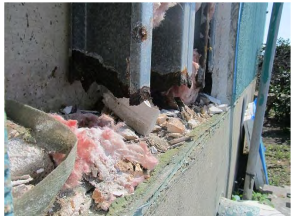
Photo #10 DTO #3 - Total member loss of sill track and bottom of vertical framing members.
