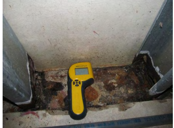
Photo #20 Moisture probe reading on exterior gypsum sheathing (0.9%) during spray testing referenced in previous photo. Water was also felt on bottom sill.
