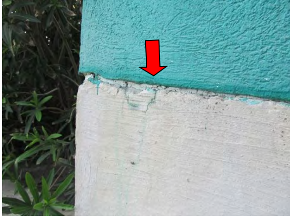
Photo #31 Deteriorated sealant between EIFS termination and foundation, typical condition throughout.
