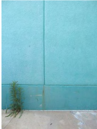
Photo #37 Staining at EIFS joint.
