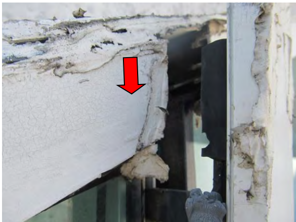
Photo #77 Detail view of displaced mullion. Note sealant in poor condition.
