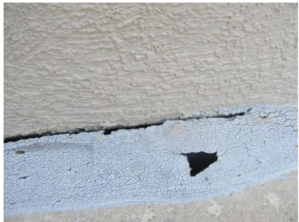
Photo #40 Detail view of typical deterioration and sealant adhesion failure at bottom of EIFS wall.
