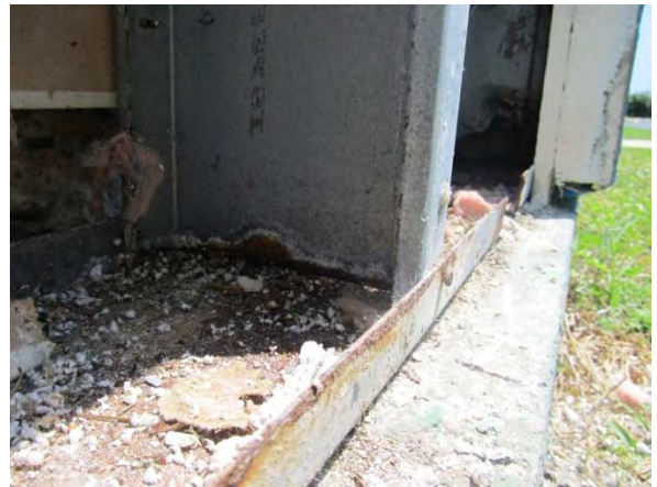
Photo #22 DTO #7 – Minor corrosion of sill track and new vertical framing member.
