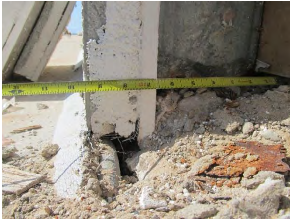
Photo #15 DTO #5 – Significant corrosion along base of wall.
