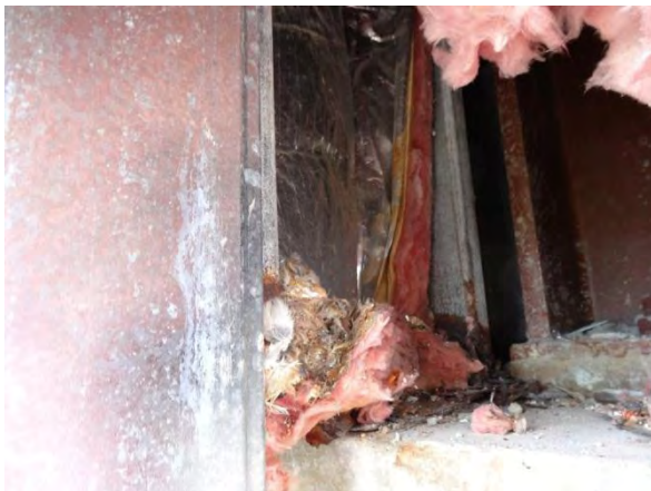
Photo #9 Moisture impacted insulation during spray testing.
