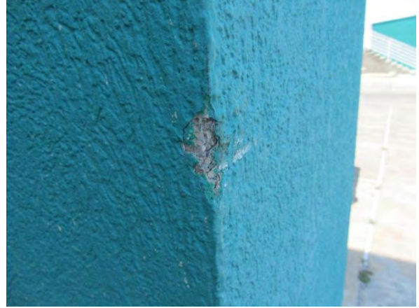
Photo #32 Damaged EIFS at corner of building.
