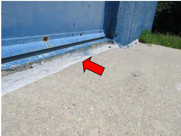
Photo #57 Detail view of deteriorated sealant referenced in previous photograph.
