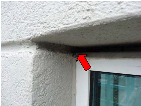
Photo #5 Opening at window corner, typical condition.
