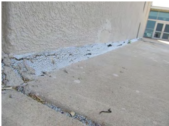
Photo #39 Deteriorated and weathered sealant joint at bottom of EIFS wall, typical condition throughout.
