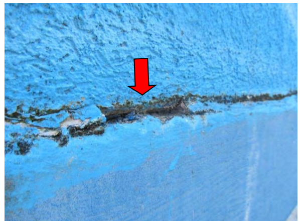
Photo #66 Detail view of typical sealant deterioration along bottom of EIFS wall.
