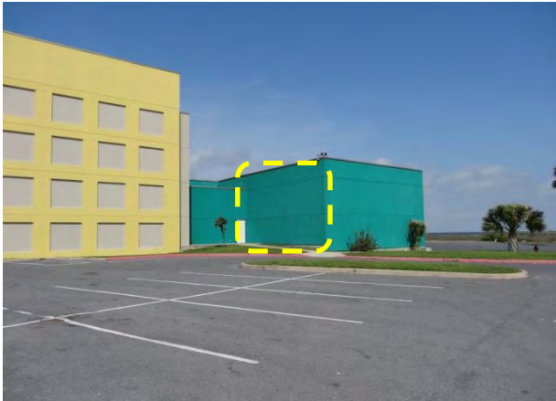
Photo #18 Green room (602) where highlighted portion of wall was reportedly blown out during Hurricane Dolly and replaced.
