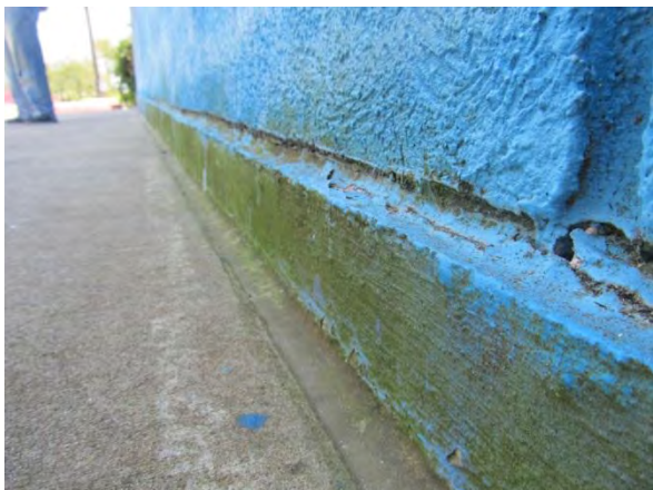
Photo #65 Detail view of sealant deterioration along bottom of EIFS wall.
