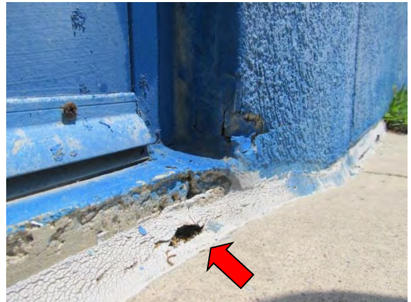
Photo #58 Hole in sealant. Also note damaged EIFS at corner.
