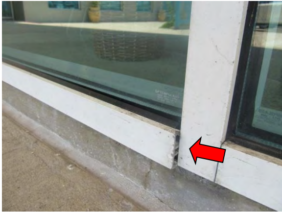
Photo #9 Displaced window framing member.
