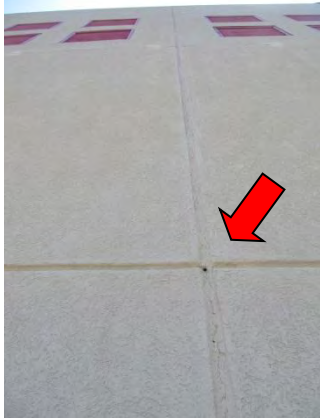
Photo #43 Deteriorated vertical control joint sealant at EIFS wall.
