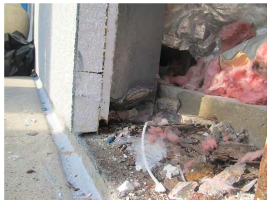
Photo #18 DTO #6 Corroded sill track and bottom of vertical framing member.
