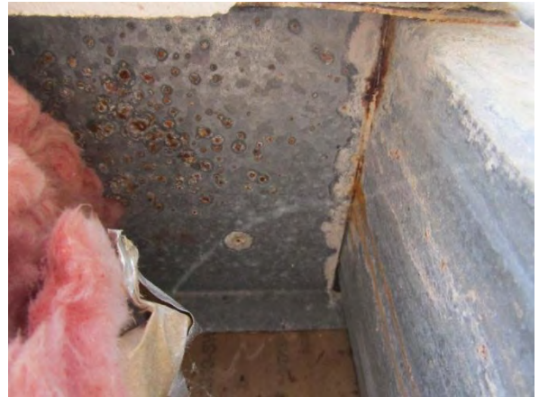
Photo #14 DTO #4 – Corrosion on window sill as observed looking up wall.
