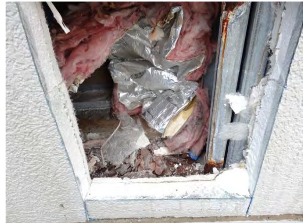
Photo #4 Water observed migrating into wall assembly.
