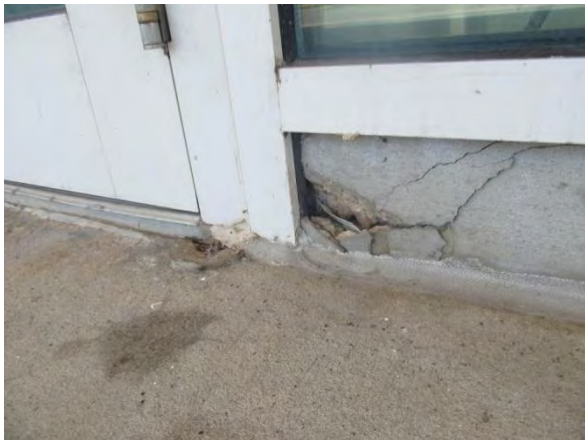
Photo #11 Detail view of spalled concrete near door referenced in previous photograph.
