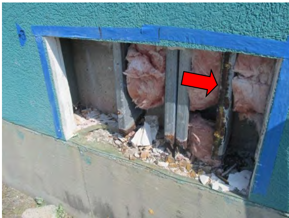
Photo #9 DTO #3 – Typical corrosion along bottom sill track and vertical framing members. Note corrosion on vertical framing member believed to be impacted from water infiltration from windows above.
