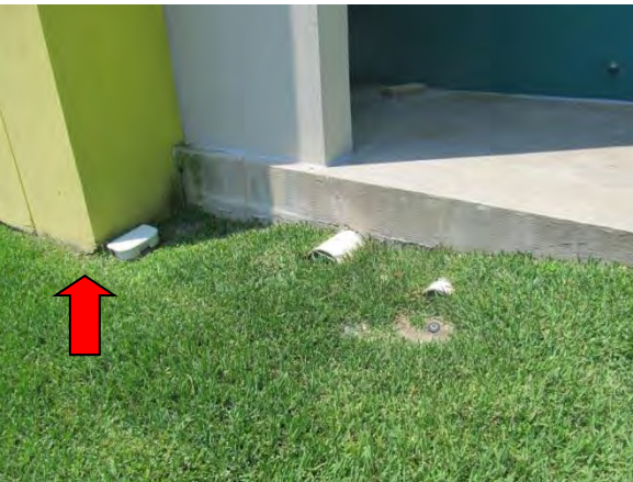
Photo #17 EIFS extends below landscaped area at northeast corner. Note piping covered by landscaping.
