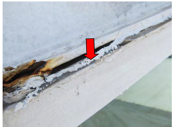
Photo #78 Typical sealant failure at window/metal flashing interface.
