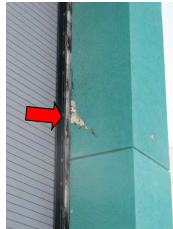
Photo #30 Detail view of damaged EIFS.
