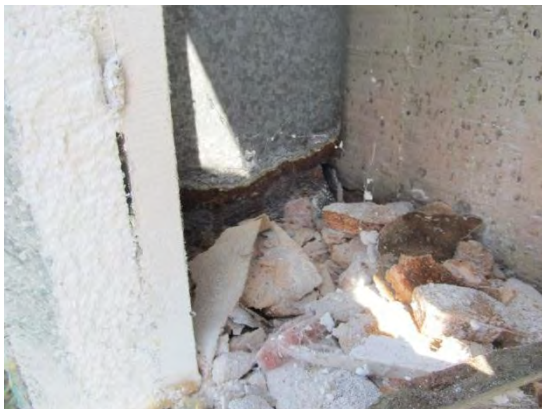
Photo #11 DTO #3 - Member loss of bottom sill track and vertical framing member.
