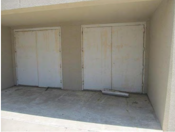
Photo #13 Entrance doors to Room 600. Facility personnel reported active water leaks under thresholds.
