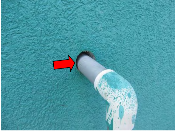
Photo #25 Unsealed pipe penetration on north wall.
