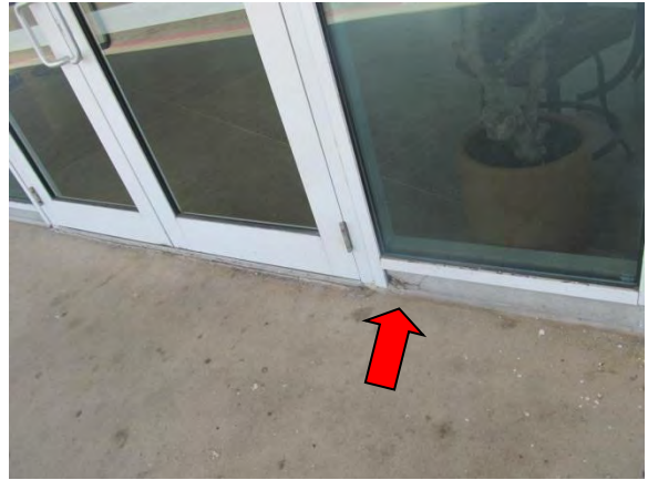
Photo #10 Spalled concrete near door.
