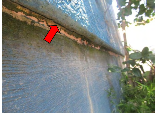
Photo #62 Sealant adhesion failure along bottom of EIFS termination, typical condition. Also note staining on sealant.
