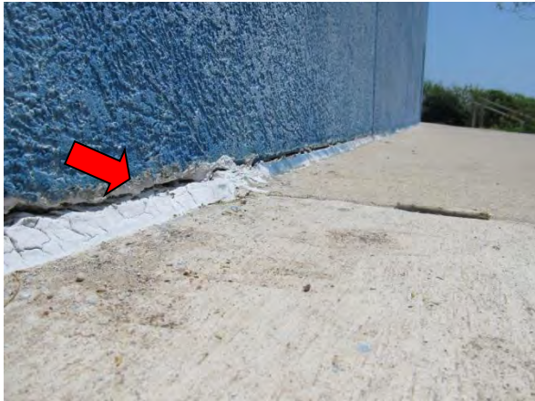
Photo #55 Sealant adhesion failure at bottom of EIFS wall, typical condition throughout.
