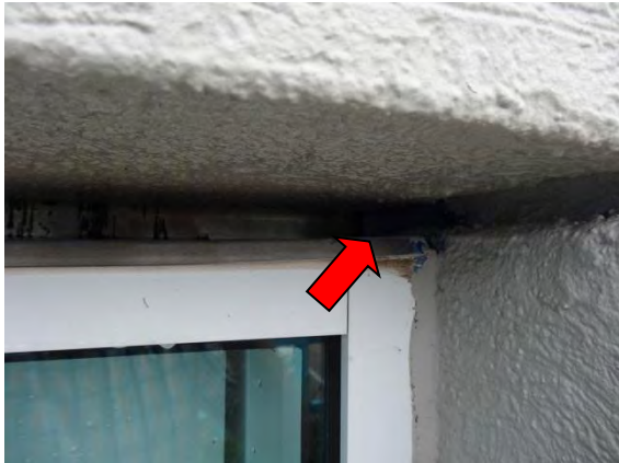
Photo #3 Typical window head flashing detail. Note metal head flashing above window and openings at corner.
