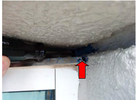
Photo #4 Detail view of opening at corner of window, typical condition.
