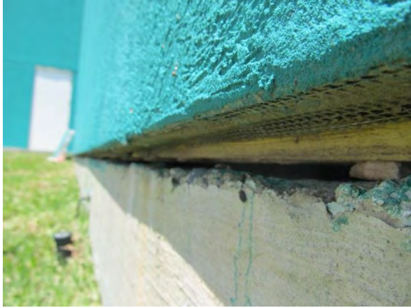
Photo #19 Exposed backwrapping and exterior sheathing at bottom of EIFS wall due to missing sealant and backer rod joint along south wall of Green Room.
