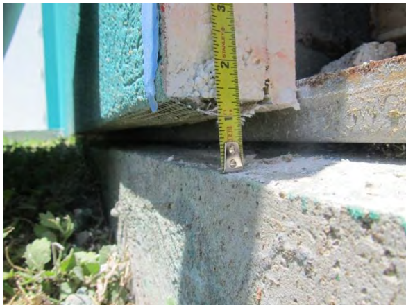
Photo #23 DTO #7 – Improper EIFS termination at foundation. Note exposed backwrapping and missing sealant joint.
