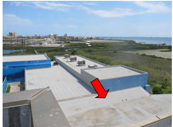
Photo #68 Overview of roof areas facing south. Note staining on lower roof over lobby.
