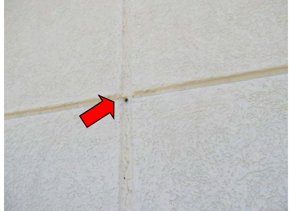
Photo #44 Detail view of hole in sealant and sealant cohesion failure in at EIFS wall.
