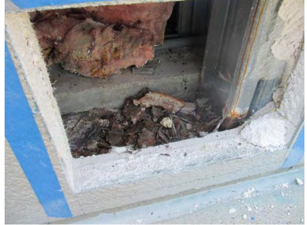
Photo #2 DTO #1 – Corroded sill track with total loss.
