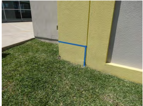
Photo #16 EIFS wall extends approximately 12" below landscaped area at the southeast corner.
