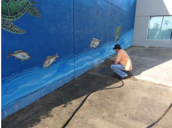
Photo #19 Water spray testing along bottom of EIFS joint on exterior "WyLand" wall.
