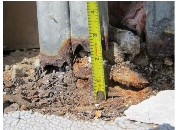
Photo #16 DTO #5 - Corrosion along bottom sill track and vertical framing members.
