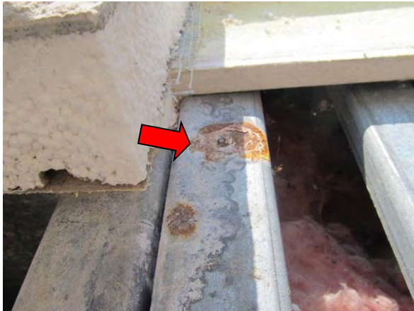
Photo #13 DTO #4 – Minor corrosion at fastener.
