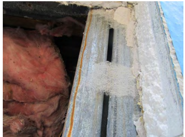
Photo #4 DTO #1 – Water stains on vertical framing member from window above.
