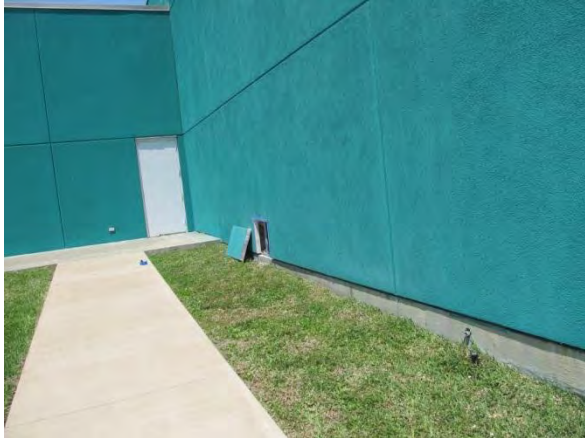
Photo #19 DTO #7 – Taken on south wall of “Green Room” on east elevation.
