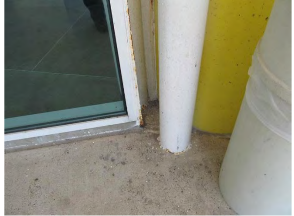
Photo #8 Deteriorated sealant joint along bottom of window frame and localized corrosion on framing members.
