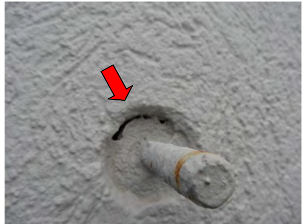
Photo #6 Opening at penetration above windows, typical condition.
