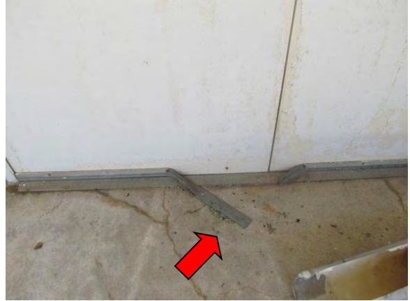
Photo #14 Detail view of damaged threshold and door sweeps.
