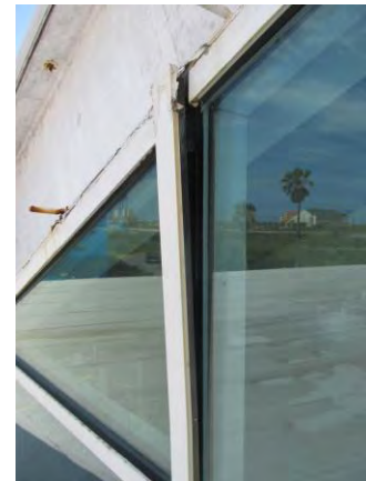
Photo #76 Displaced vertical mullion.
