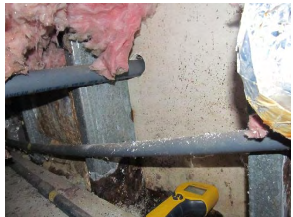
Photo #18 Moisture probe reading of exterior gypsum sheathing (4.9%). Dampness was felt during spray testing referenced in previous photographs.
