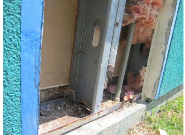
Photo #20 DTO #7 – Minor corrosion along replaced sill track and vertical framing members.
