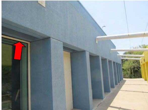
Photo #51 Openings along window heads are unsealed.
