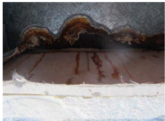
Photo #6 Bottom of sill. Water stains along interior sheathing.
