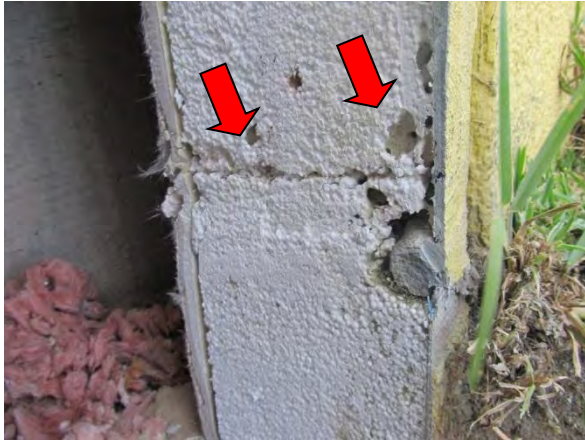
Photo #7 DTO #2 – Evidence of insect infestation in EPS insulation.
