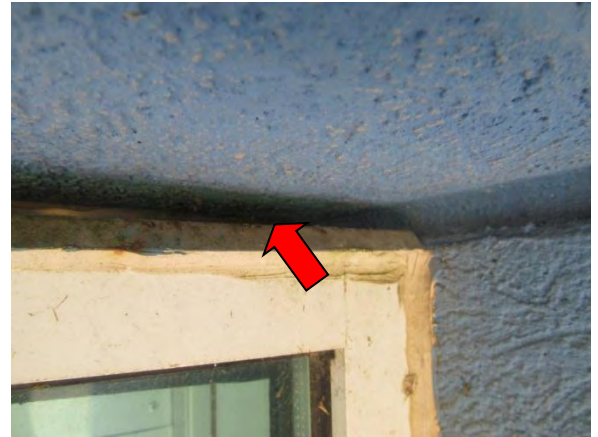
Photo #52 Detail view of unsealed window head.
