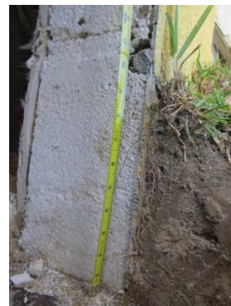
Photo #6 DTO #2 – Part of the EIFS extending 12" below grade.
