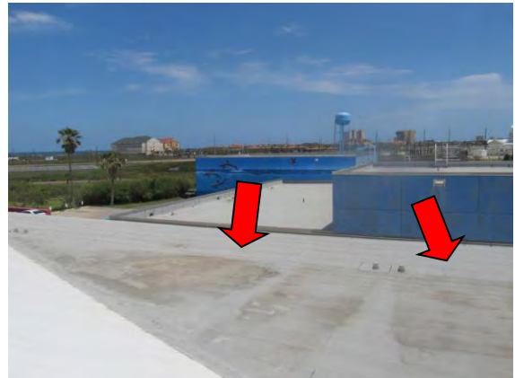
Photo #70 Staining on capsheet membrane due to ponding conditions from inadequate roof slope.
