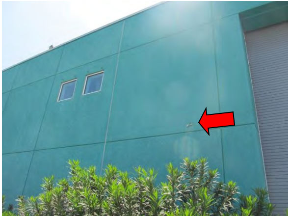
Photo #27 North elevation. Displaced/damaged wall penetration exposing EIFS reinforcement.
