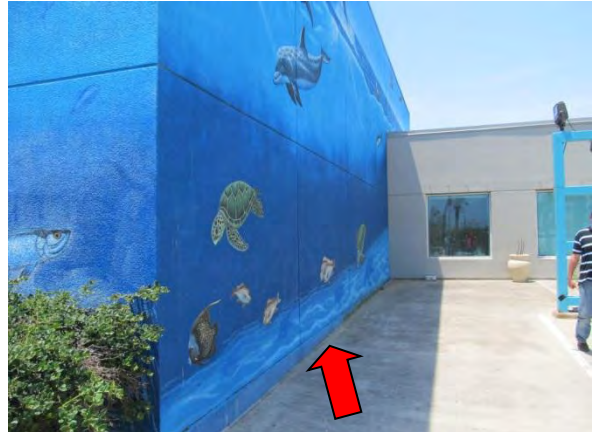
Photo #64 Sealant deterioration along north "WyLand" wall, typical condition.
