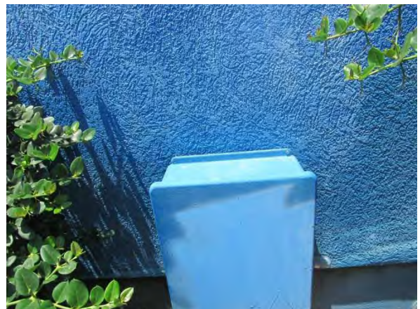
Photo #60 Electrical box along east wall.
