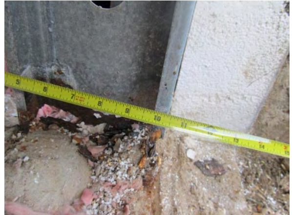
Photo #8 DTO #3 – Corrosion along bottom of vertical framing member. Sill track was completely corroded.
