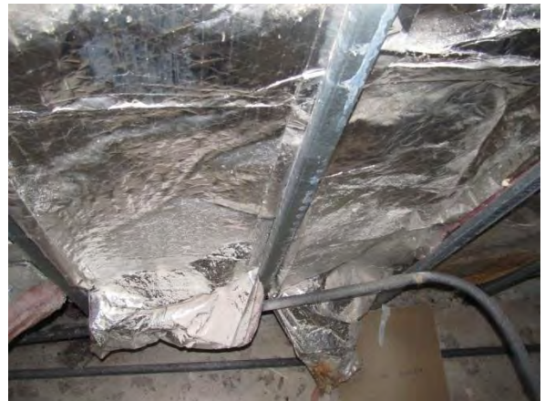
Photo #24 Interior opening approximately 6' above Opening #10. No evidence of distress or moisture impacted materials were observed.
