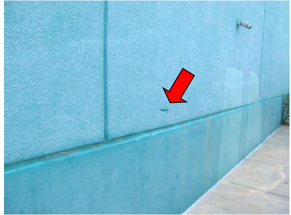
Photo #34 Damaged EIFS adjacent to Receiving area.
