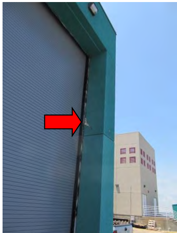
Photo #29 Damaged EIFS near overhead door.
