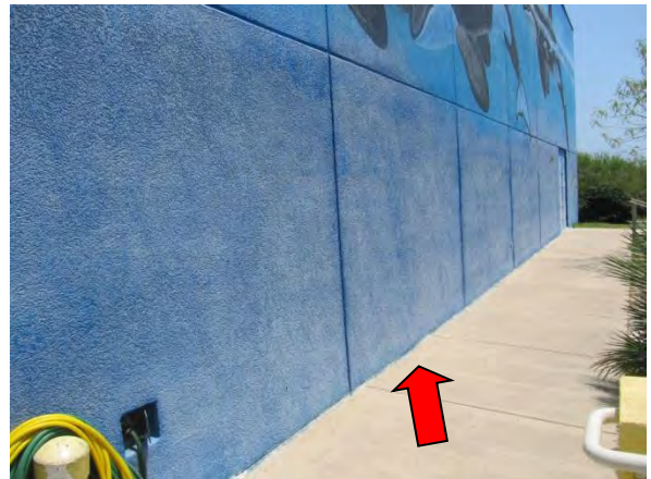
Photo #54 Deteriorated sealant at bottom of EIFS wall.
