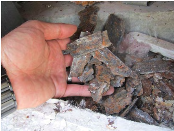
Photo #3 DTO #1 – Corrosion scale along sill track.
