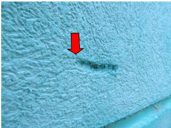
Photo #35 Detail view of damaged EIFS referenced in previous photograph.
