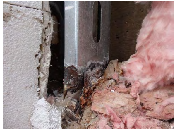
Photo #10 Moisture impacted insulation and corrosion on vertical framing members.
