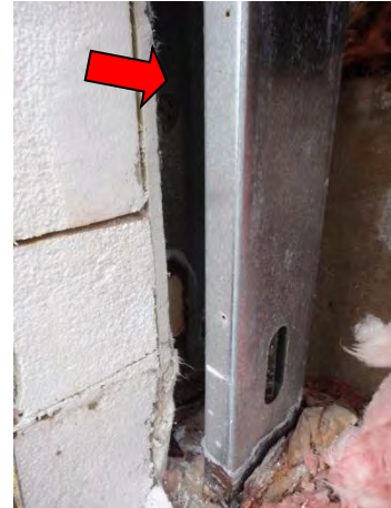
Photo #8 Water observed migrating along EIFS termination and continuing down floor line.
