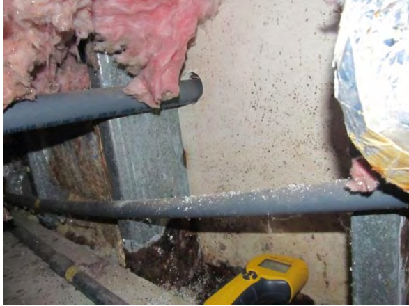
Photo #61 Interior view of conduit penetration from electrical box. Water was observed migrating through opening during water spray testing.
