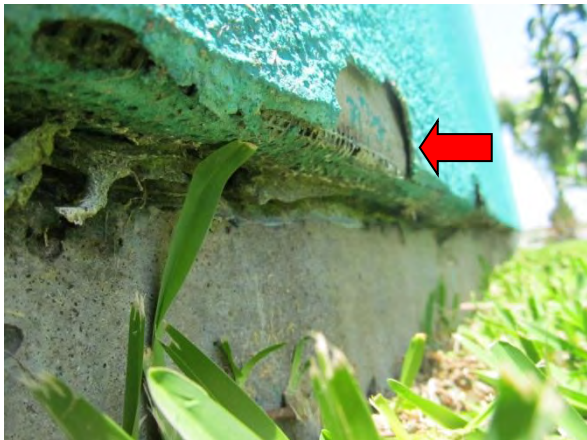
Photo #23 Exposed backwrapping along bottom of EIFS wall. Note spalled EIFS finish coat.
