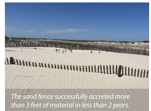
Adaptive management for foredune restoration that included native hay installation, bare-root planting, and sand fence installation
